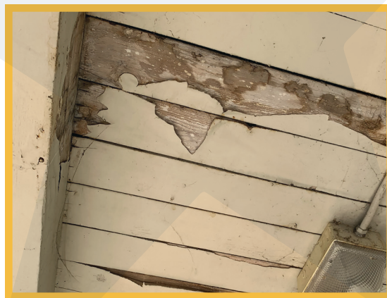
DAMAGED ROOF AT CULVER CITY MIDDLE SCHOOL
