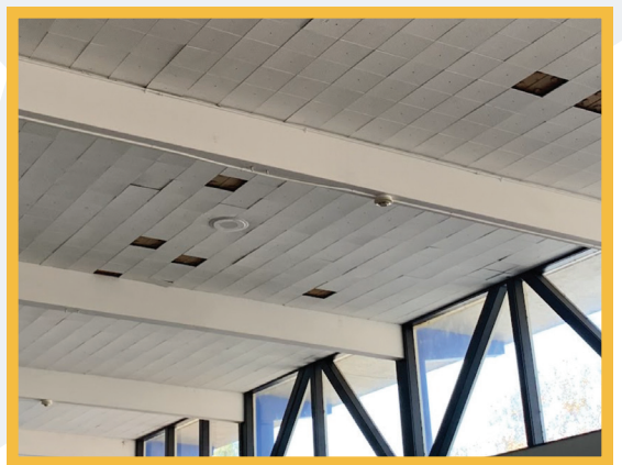
FALLING CEILING TILES AT CULVER CITY MIDDLE SCHOOL
