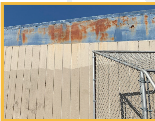
DETERIORATED ROOF AND CLASSROOM BUILDING AT CULVER CITY HIGH SCHOOL
